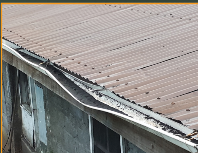
Ash loading can cause gutters to partially or completely detach from buildings. Basaltic ash from 2018 eruption of Ambae volcano, Vanuatu. Photo credit: Sally Dellow, GNS Science.
