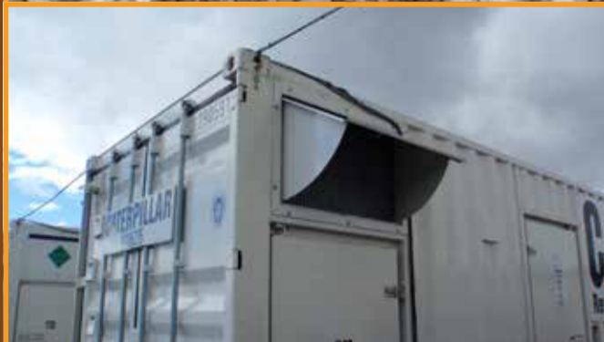
Adaptations to protect generator equipment in Bariloche, Argentina, from repeated airborne ash exposure following 2011 eruption of Cordón Caulle volcano, Chile. Top: sealed fuel valve. Bottom: hood to protect air intake. Photos: Tom Wilson.
