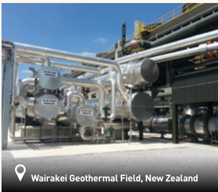
Mercury Energy geothermal power station
