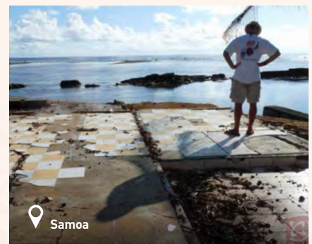
Samoa Viewing coastal tsunami damage
