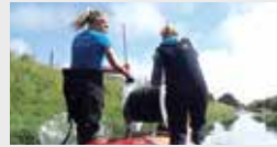
P2 Laying fibre optic cable to analyse groundwater-surface water interaction – Abigail Lovett
