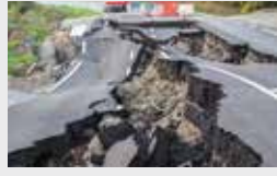
P32 Hundalee Fault rupture as it crosses SH1 – unknown
