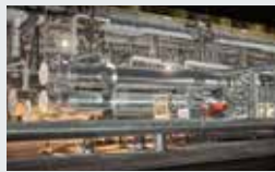
P33 Ngatamariki Power Station – Chris Sisarich
