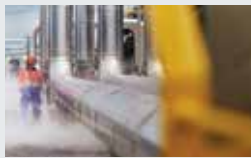
P32 Ngatamariki Power Station – Chris Sisarich
